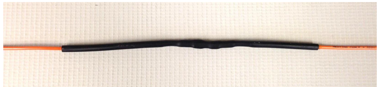
23) Finally slide the long Black sleeve so it is centrally over the repair and heat shrink in position. Allow the sleeving to cool down and check the resistance and insulation resistance between the live wires.
